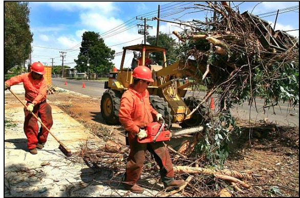
Men at Work: A work crew clears debris from trees that are being removed from Gibbs Park in Huntington Beach. (Mark Martinez, The Orange County Register)
